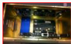
Power Control Unit (PCU)
